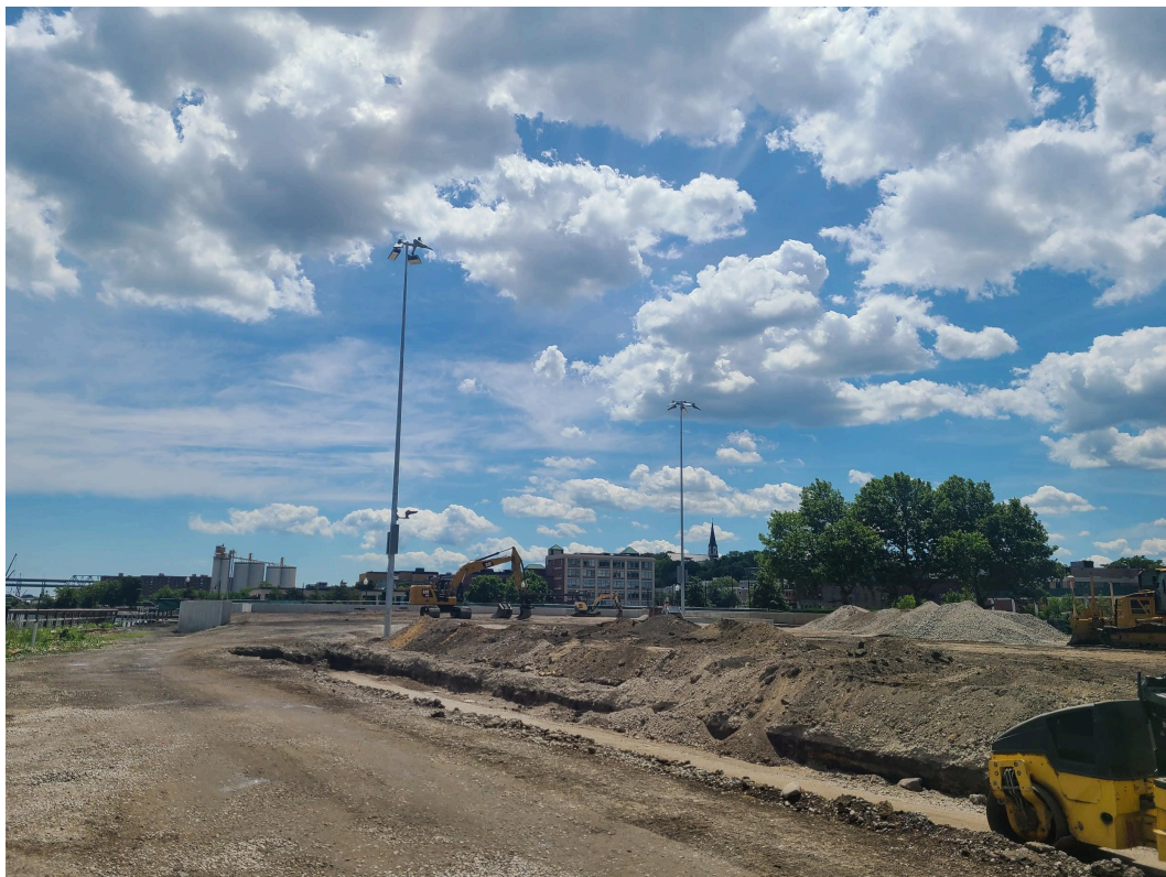
New light poles by the Schrafft's corner, and you can start to see the new higher elevation of the ballfield taking form. (The trench in the foreground is where fill will be added, and the new berm will be located.)
