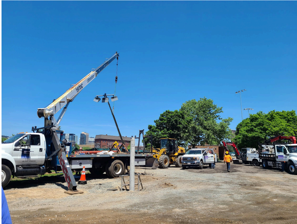
A new light pole dangles from the crane that will guide it into place on the base in the foreground. Installed light poles are visible in the distance, where the ballfields are located.
