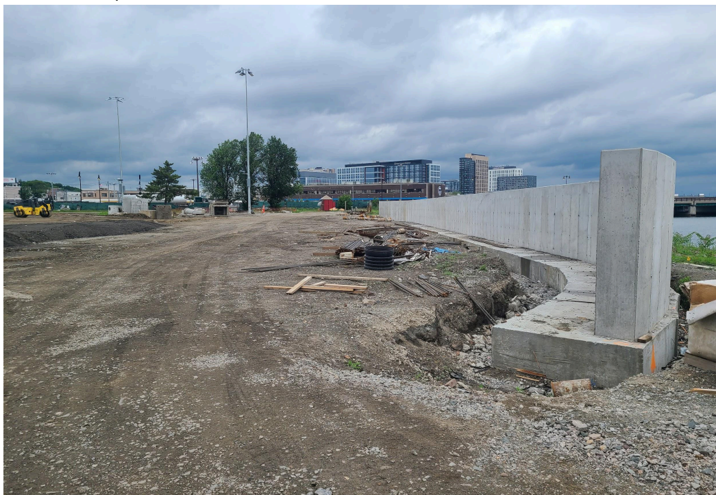
A new concrete retaining wall to support the part of the berm with the playground and splash pad on top of it.
