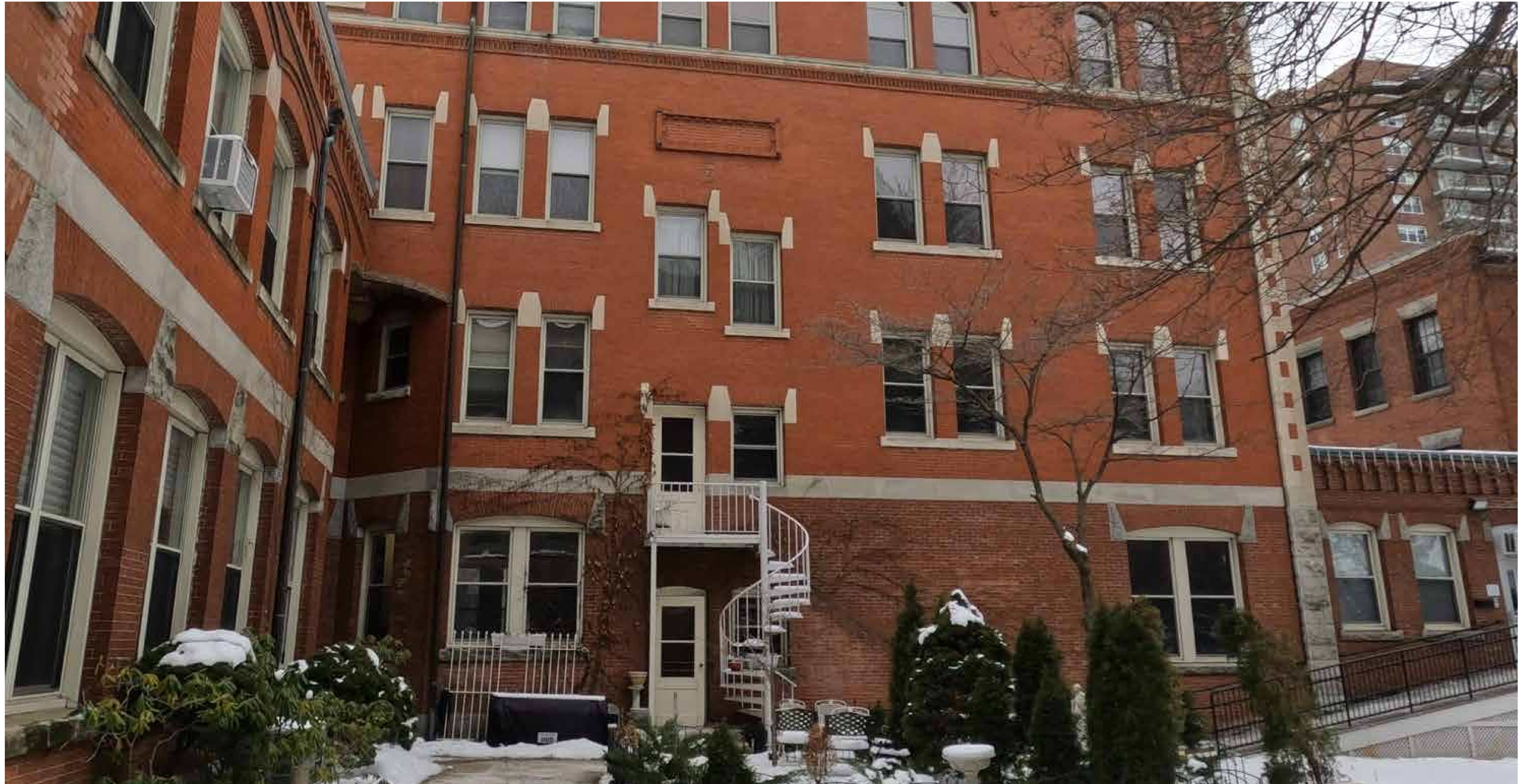
NORTH RECTORY FACADE & STAIR CONDITION [COURTYARD VIEW]
