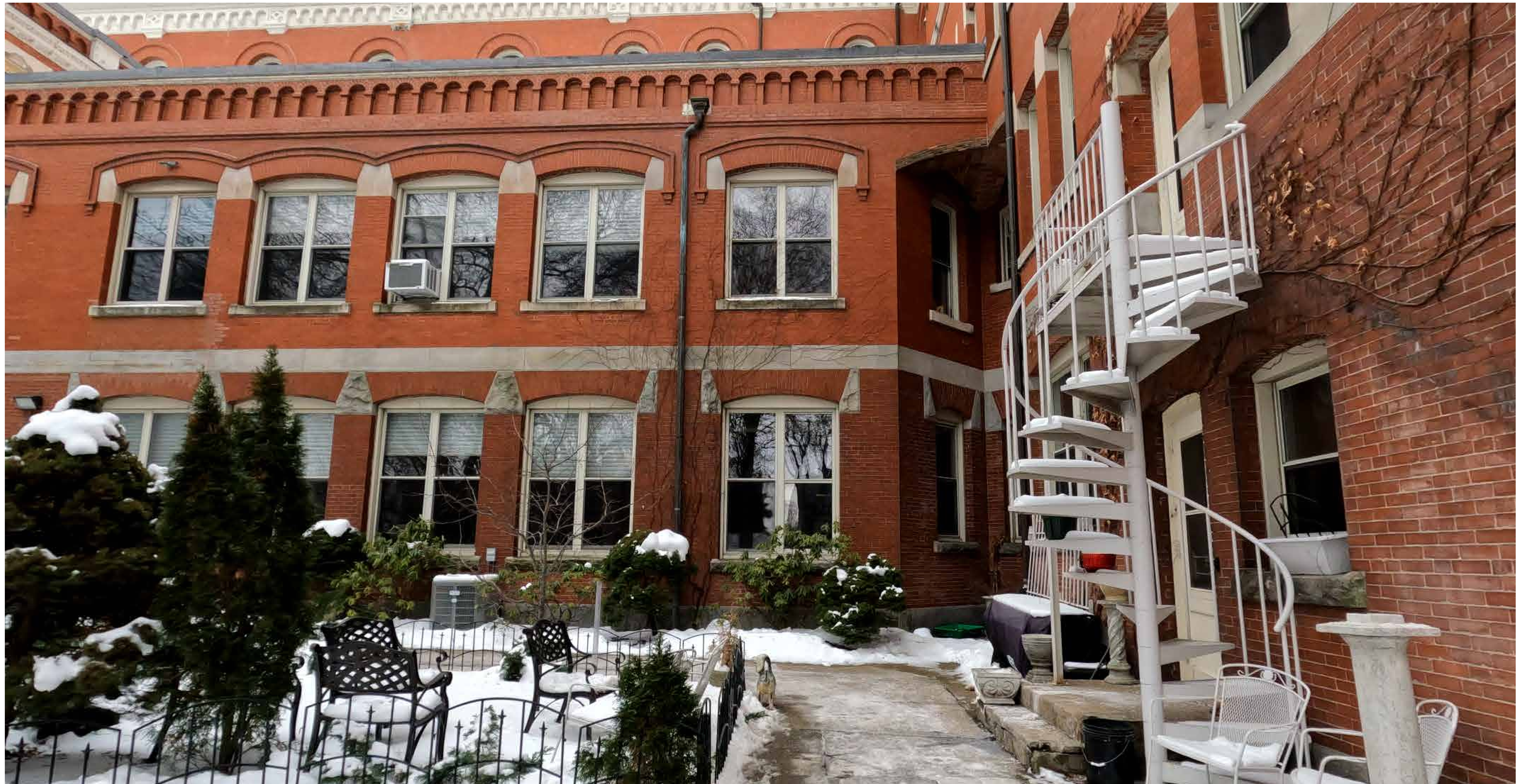
NORTH RECTORY FACADE & STAIR CONDITION [COURTYARD VIEW]
