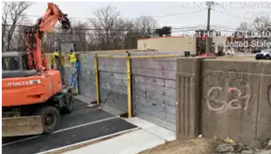
Figure 5 – Stop Log Example (Photo Courtesy of East Hartford, CT)
