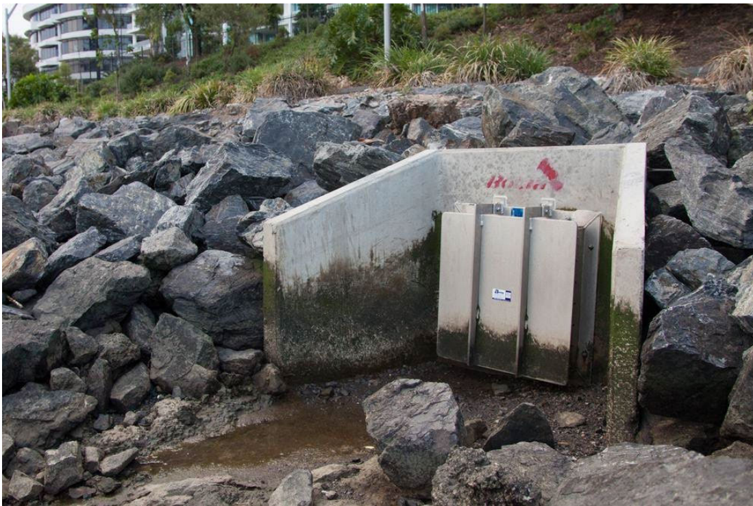
Figure 9: Example of Flap Gate Style Check Valve (Photo courtesy of USACE Norfolk District)
