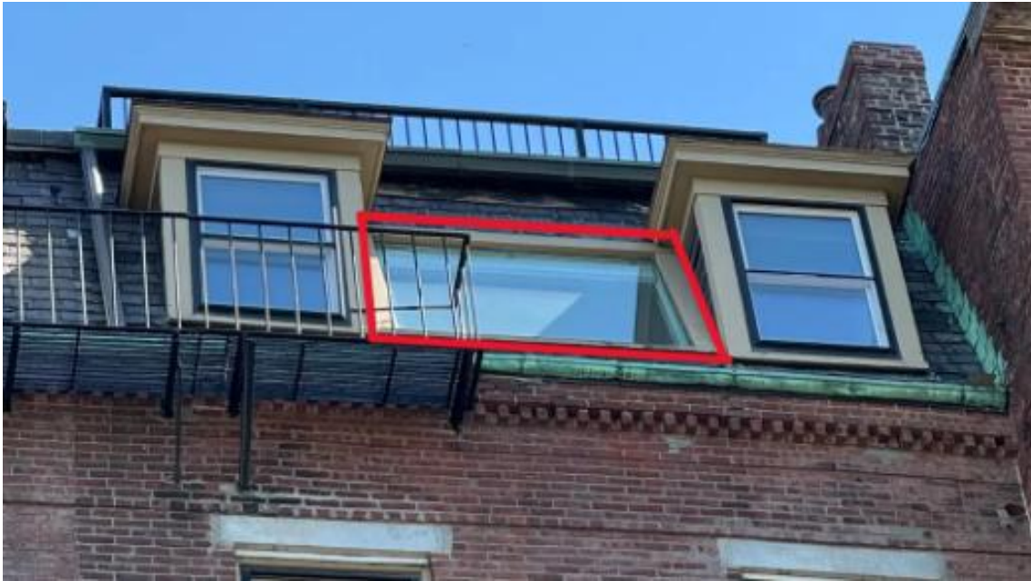
EXISTING ESTATICARY WINDOW WITH EXTERIOR ROTTED FRAME
